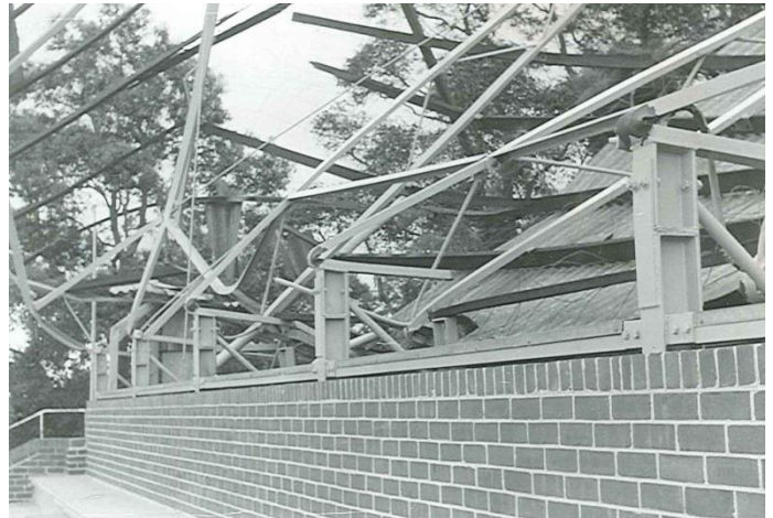
Storm damage to grandstand 1965.
